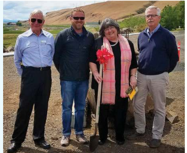
Groundbreaking for West Side Landscaping May 2019 (Building and Grounds Committee and Board Project). Pictured Trustee Juris Sarins, Mike Clough, Caretaker, Colleen Schafroth Executive Director, and Ian Grabenhorst, President.
